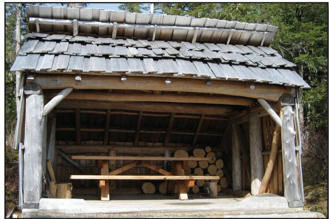
Figure 107—The entrance to the Three Lakes camp shelter at the Tongass National Forest is level with the ground.
