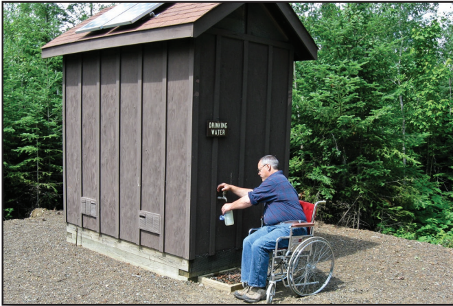
Figure 18—The water pump inside the pumphouse at Vermilion Falls Recreation Area on the Superior National Forest is powered by the solar panels on the roof. People can obtain drinking water without using a handpump at this site that has no electric service.
