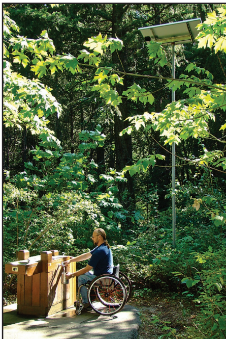
Figure 19—The water pumps for many campgrounds, such as this campground in the deep, narrow Icicle River Valley of the Okanogan-Wenatchee National Forest, can be housed in small pedestal enclosures and powered by solar panels on an adjacent pole. The pedestal enclosure also houses solar batteries.
